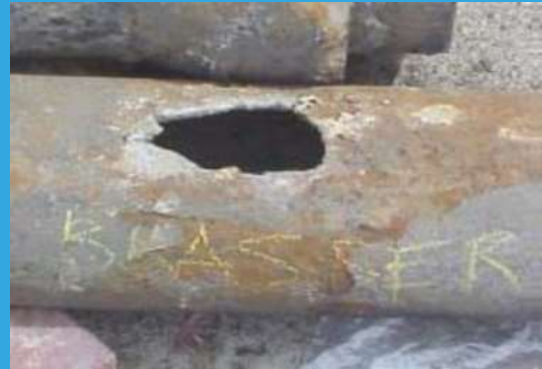
Pipe Wall Rupture
