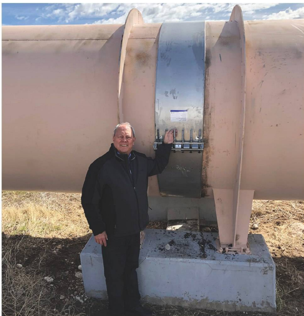
HYMAX's Denny Setzer after the HYMAX VERSA was installed on the pipe in less than one hour. All photos courtesy of HYMAX
