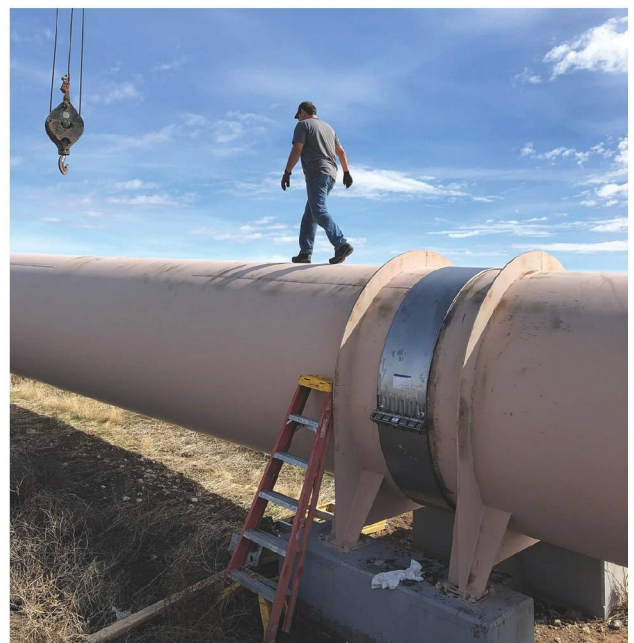
A&B Irrigation plans to save tens of thousands of dollars in labor costs and equipment rentals that would otherwise be needed to complete the project.
